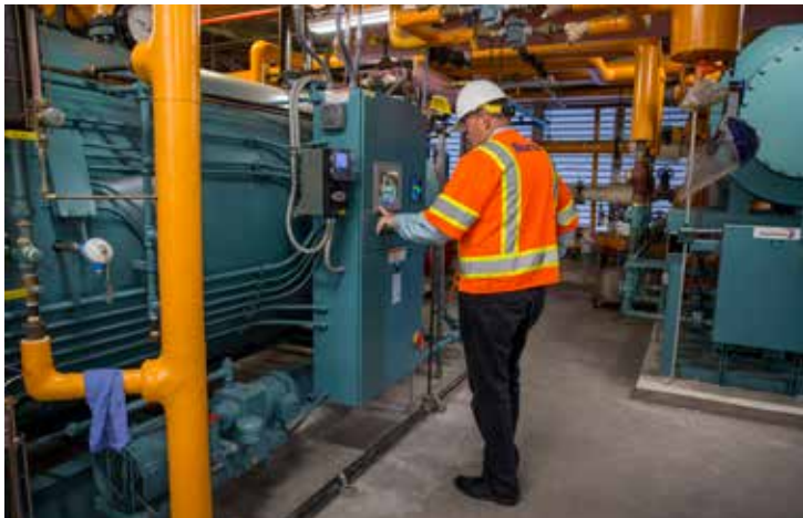
Photos: Burns Engineering
